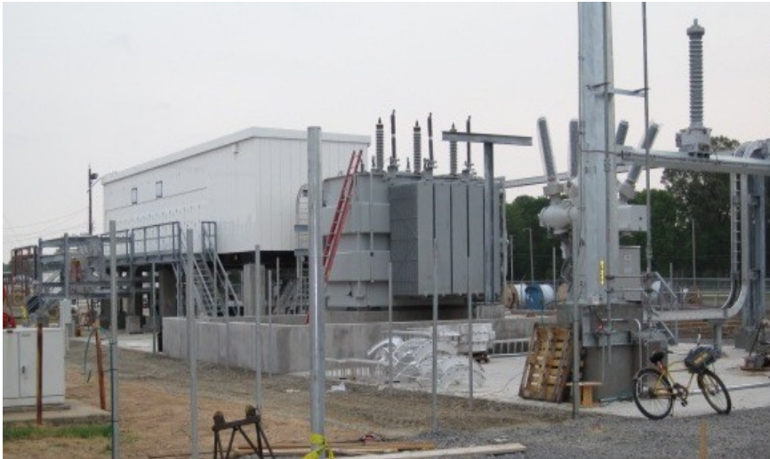
The Angus Chemical Company in Sterlington anticipates using the Retention and Modernization Tax Credit to support the installation of electrical upgrades.
